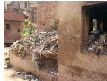
Unauthorised Garbage Dump
