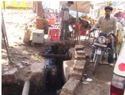
Open drain with stagnant
